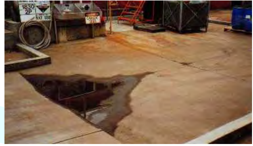
5.5 Spills of chemistry should be avoided, and cleaned up promptly.
