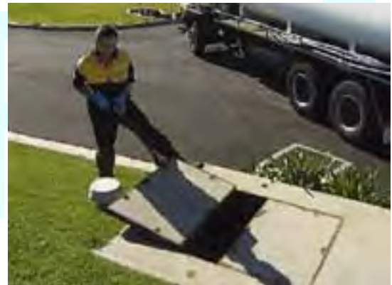
5.1 Larger operations might have their balancing tank outside.
